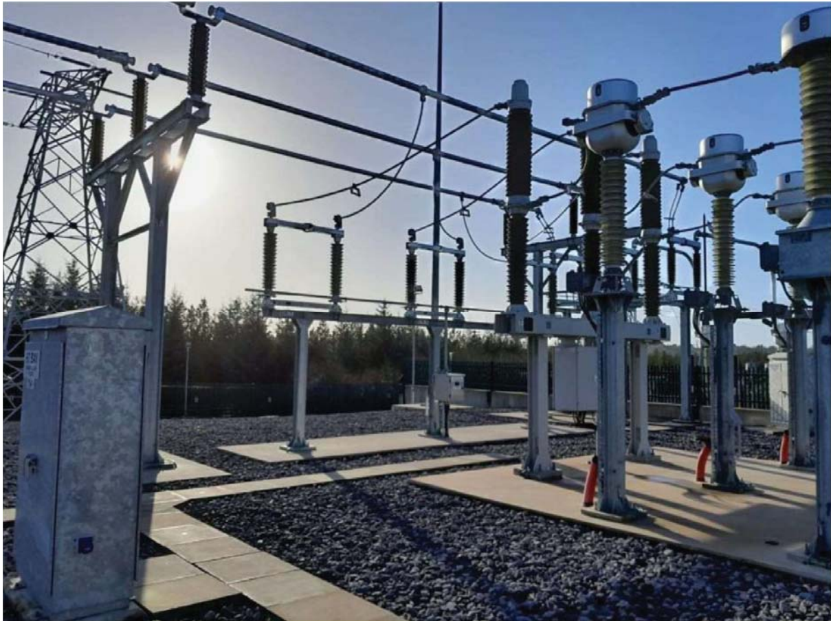
Typical 110kV Electrical Infrastructure.
