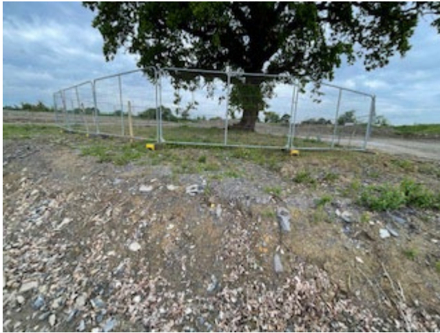
Scrub removed, ivy severed and removed, open drain backfilled and temporary protective fencing in place during enabling works.
