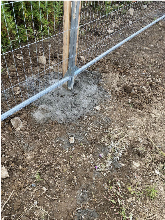
Fencing reinforced with timber stakes and concrete base in parts to ensure robustness and stability during construction phase
