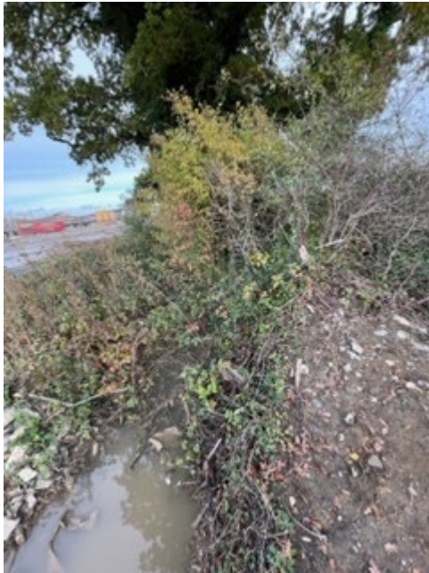
Open field drain full of stagnant water, prior to removal and backfilling.
