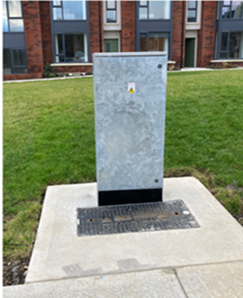
Typical ESB Meter Cabinet
