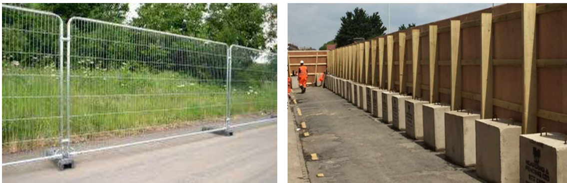
Fig 5.3 Examples – Demountable ‘Heras’ fence and solid timber hoarding with ballast blocks
