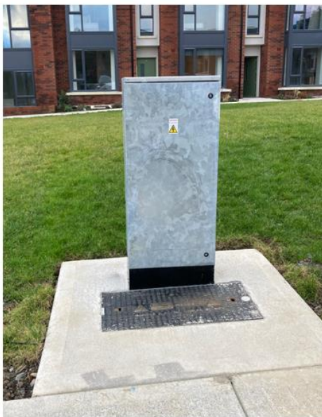
Typical ESB Meter Cabinet
