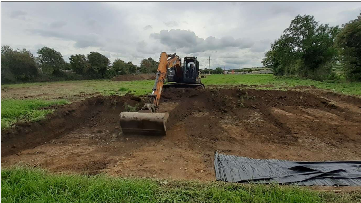
Plate 2: View of topsoil stripping uncovering the ditch in the northwest portion of the site, facing south
