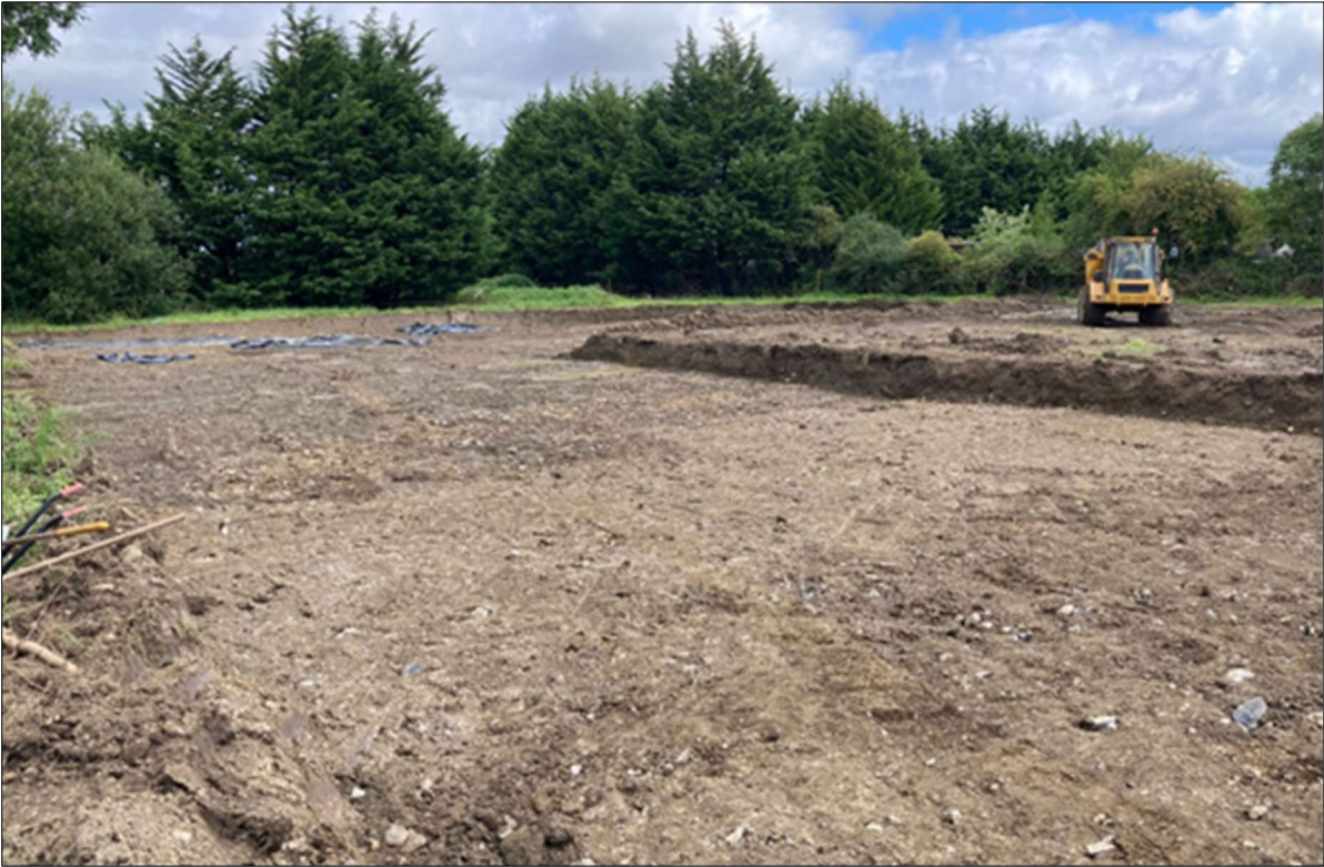
Plate 8: View facing northeast from the southwest corner of the site during topsoil stripping
