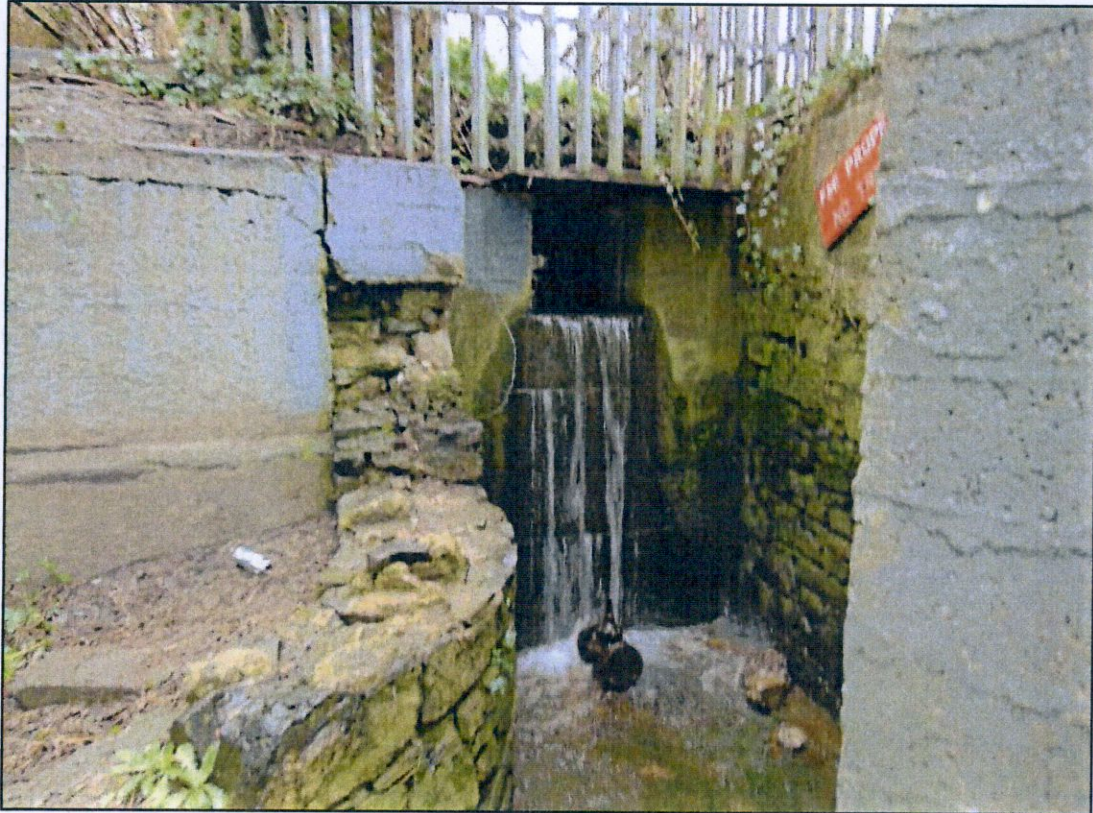
Photo 3: Concrete Tank Outlet
