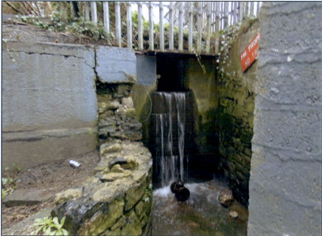
Photo 3: Concrete Tank Outlet
