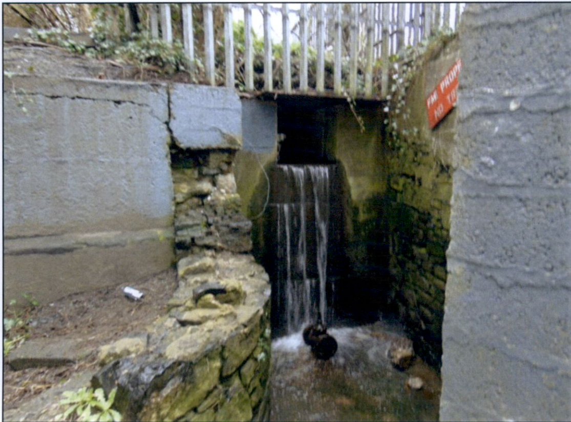
Photo 3: Concrete Tank Outlet
