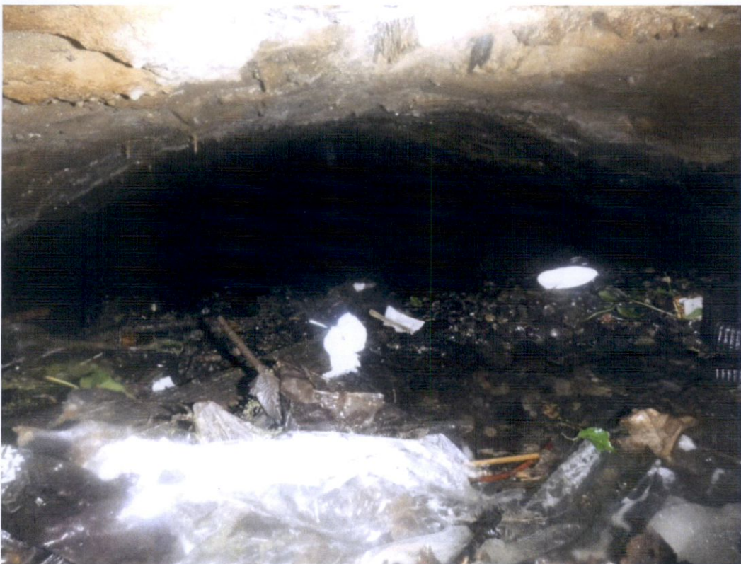
Photograph No. 2 Upstream End @ 2 m. Blockage in Arch Barrel
