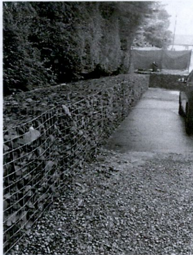
Figure 9 – Floods Defences at rear of Lismay Lodge along Bank of the River Poddle
