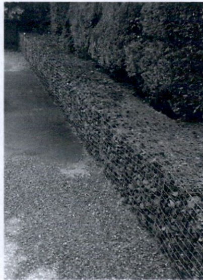
Figure 10 – Floods Defences at rear of Lismay Lodge along Bank of the River Poddle
