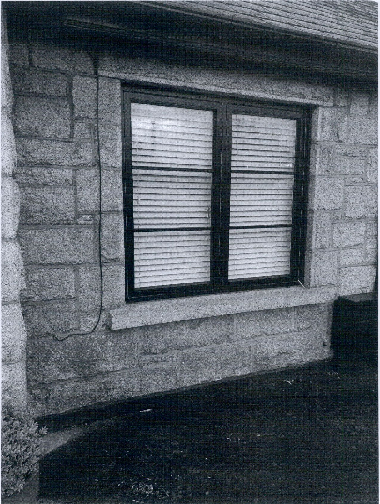
Heavy granite sills at 186 Whitehall Road, window design based on photos of original windows.
