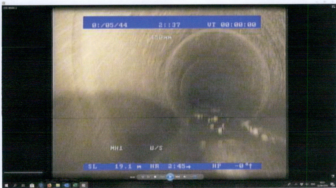
Distance 19.1m Standing water. No connections
