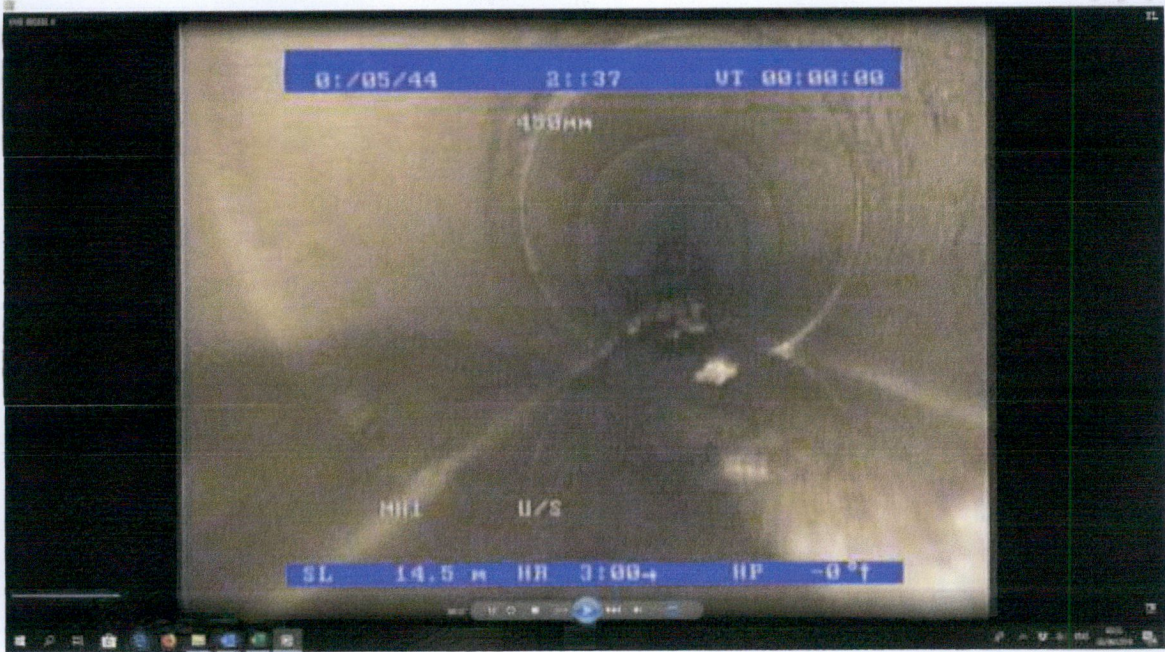
Distance 14.5m Standing water. No connections
