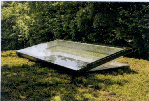
Figure 9. Image illustrating an opening Velux rooflight used to gain access for maintenance purposes to a bio-diverse type green roof
