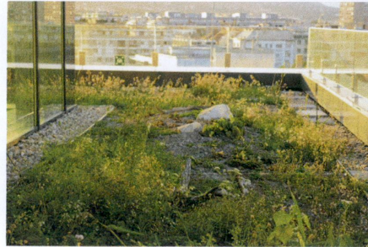
Figure 8. Image illustrating 500mm width gravel trim to the base of all walls and roof penetrations, dead log piles and small boulders on a bio-diverse semi-intensive type green roof
