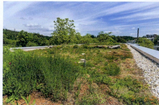
Figure 10. min. 300mm width gravel perimeter trim to roof parapet, required as a fire break under the FLL and GRO green roof guidelines
