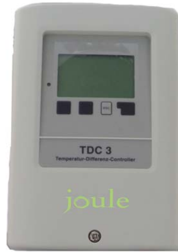
Figure 15: Joule Control Panel
