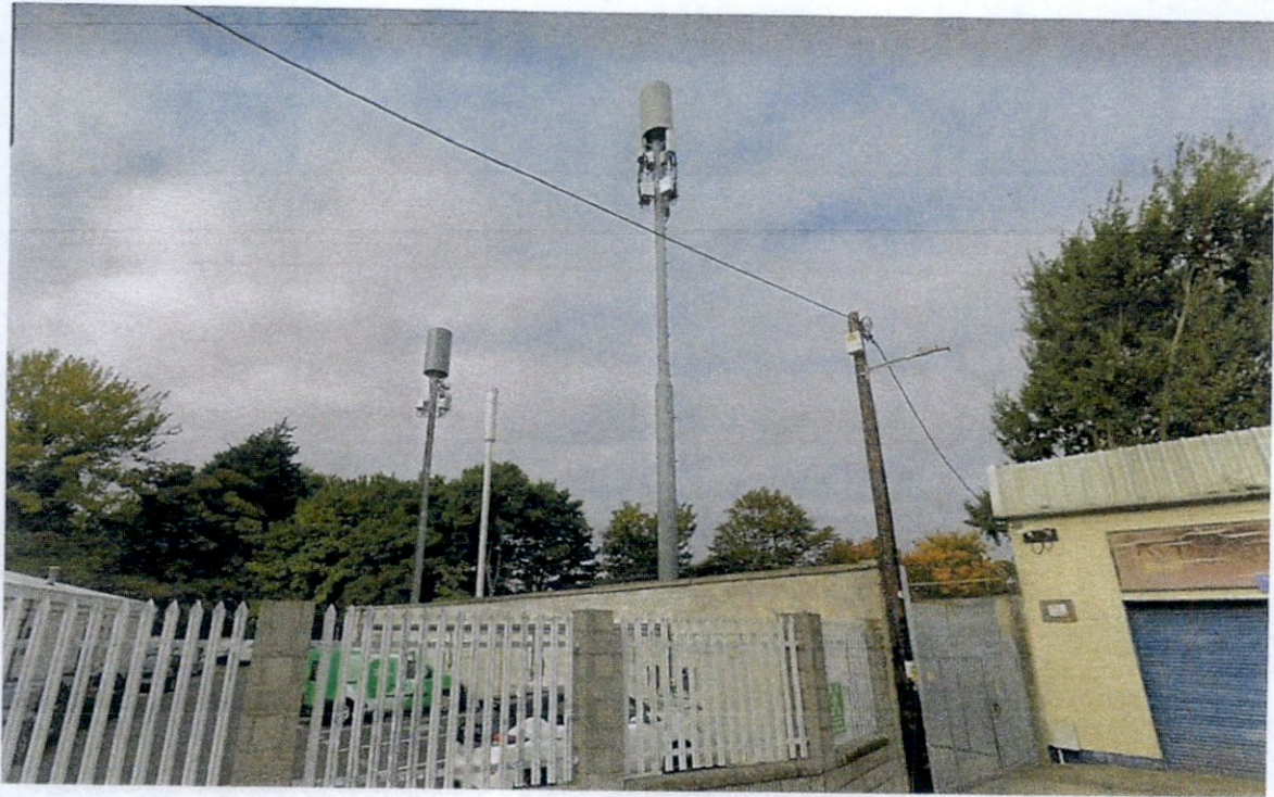
Figure 5 Existing Three Ireland, Vodafone and Eir Poles co-located at Fortfield Lane
