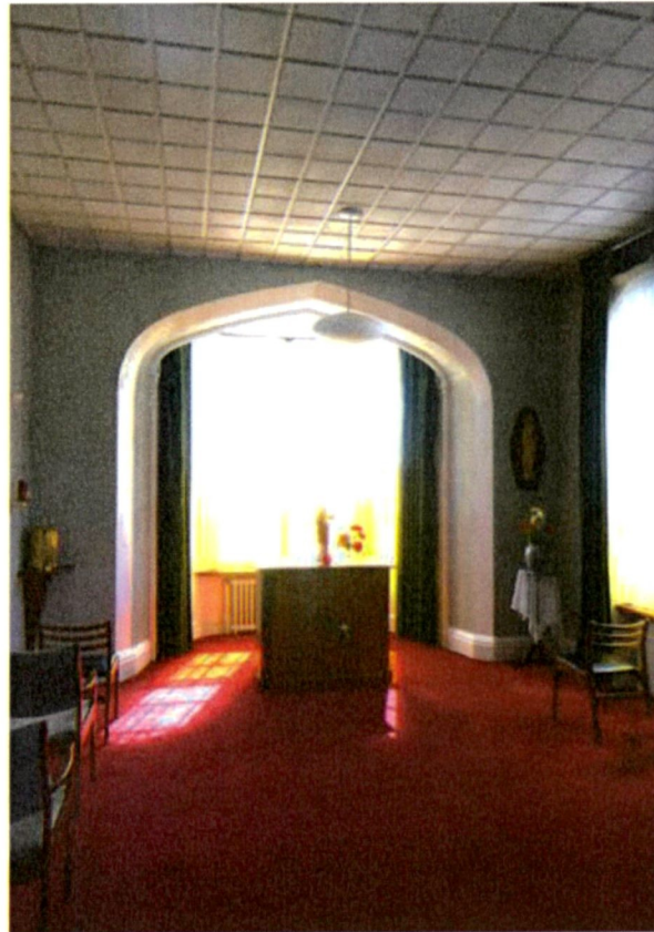
(Fig 26) View above of the former living room located at the junction of the eastern and southern wings with modern dropped ceiling and presently used as a private chapel. The room retains good window joinery, likely cornice-work above dropped ceiling and an original chimneypiece.
