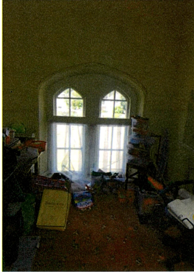
(Fig 66) - Paired neo-gothic windows within second floor of staircase tower (staircase 02) noting inserted floor cutting across windows.
