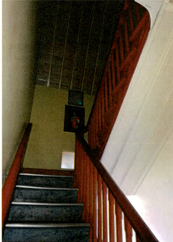
Fig 58: Staircase (01) continues to the second floor landing with continuous handrail and consistent standard and quality of joinery. Expressed joisting to underside of staircase.
