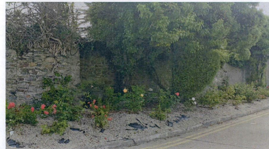
Existing 2.2m high stone wall / render mix. Note: small section of existing stone wall to be demolished and replaced, to match existing, to site entrance – refer to Landscape plan 610 for further details.
