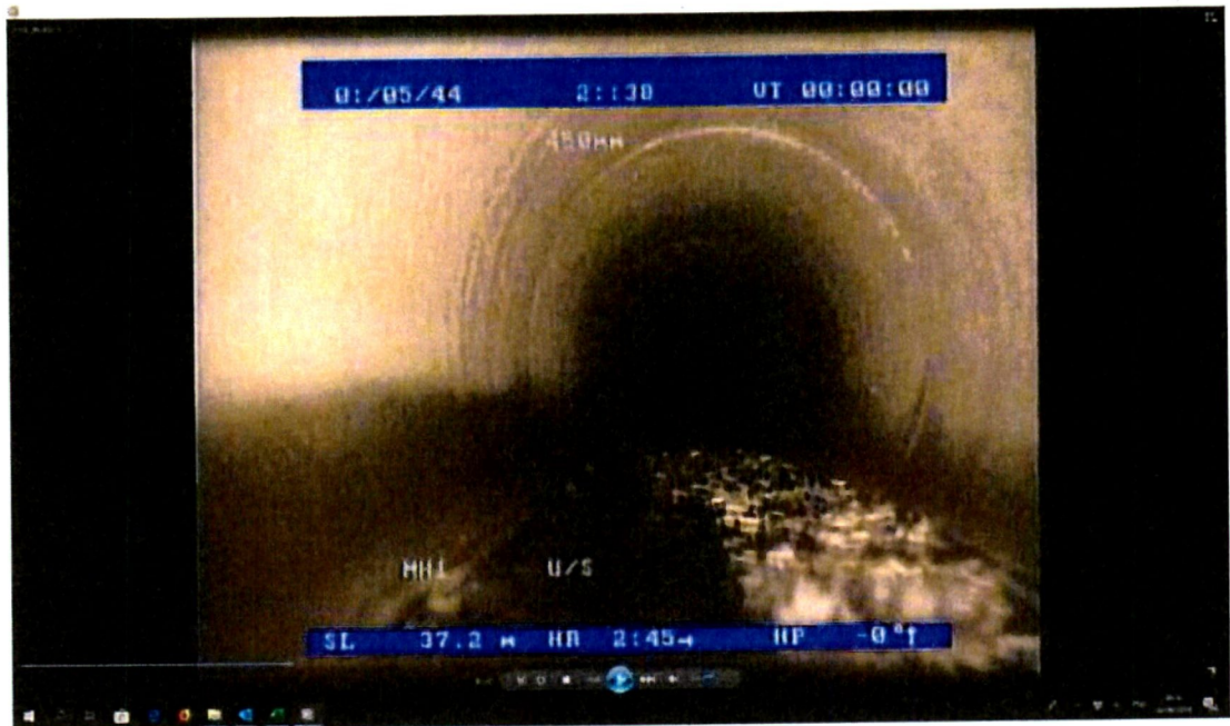
Distance 37.2m Debris in pipe. No connections
