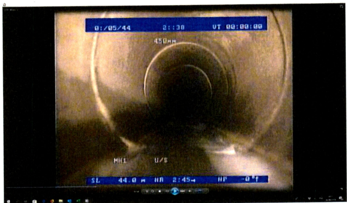
Distance 44.0m. Standing water, No connections
