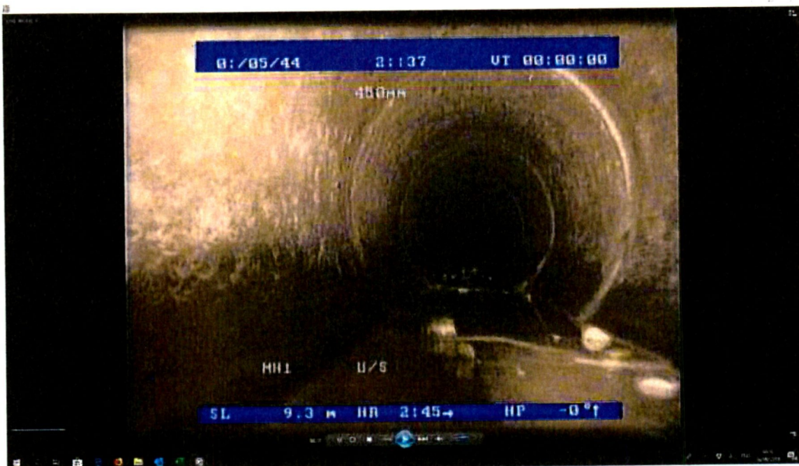
Distance 9.3m Standing water. No connections
