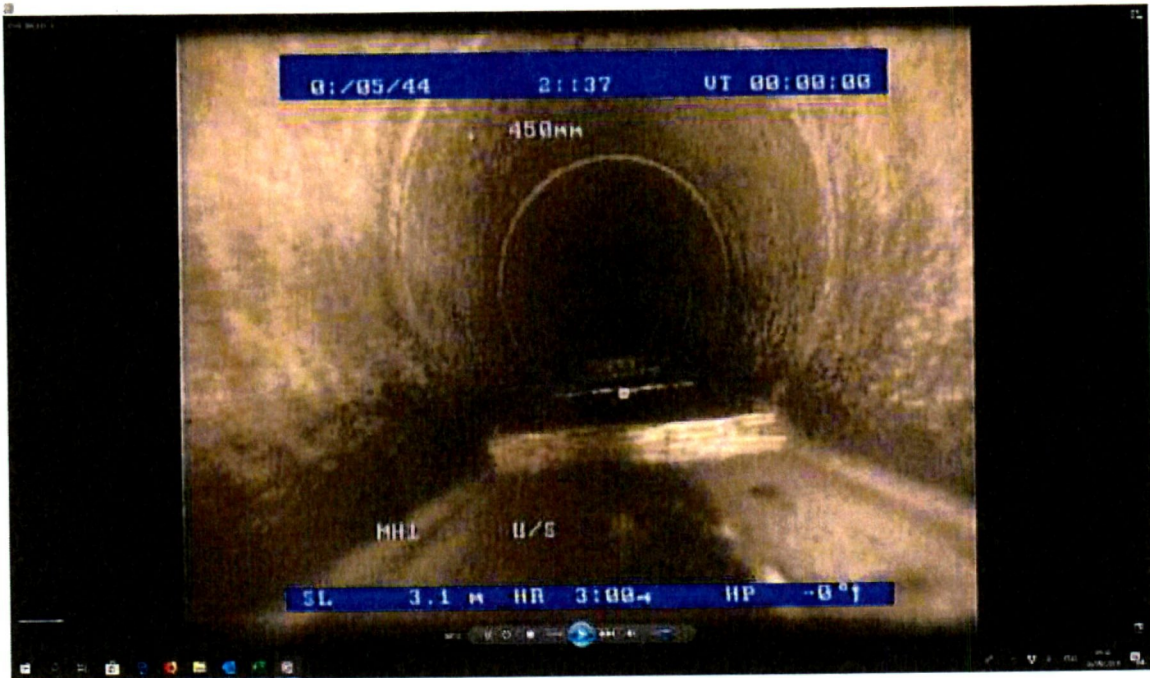
Distance 3.1m Standing water. No connection.
