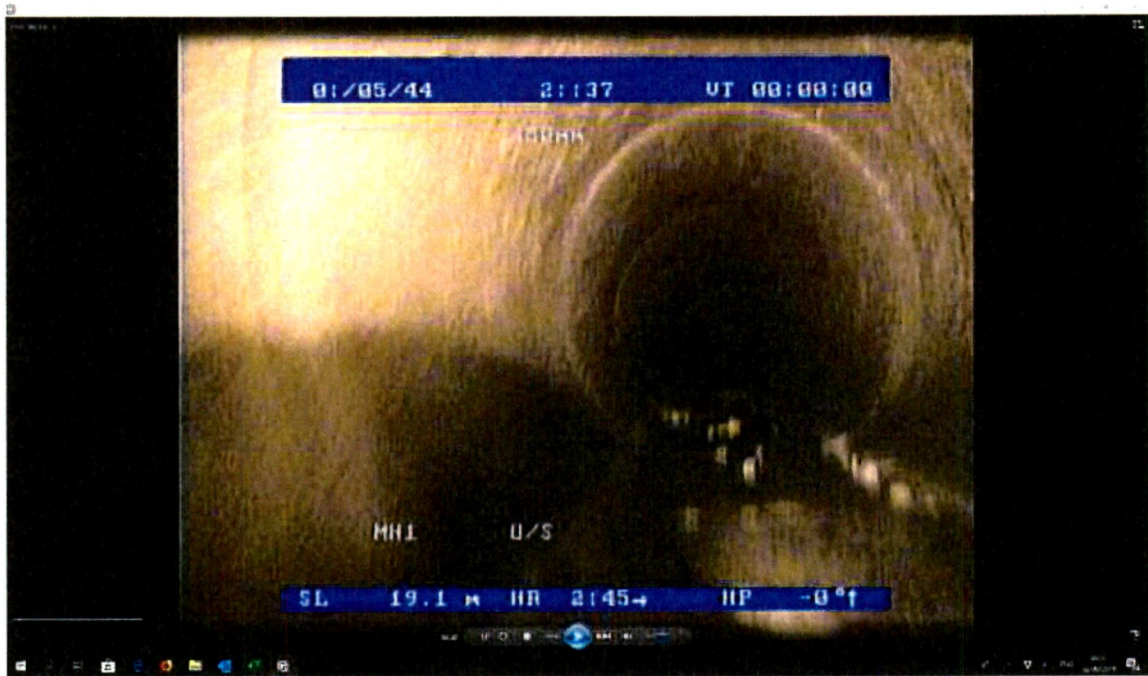
Distance 19.1m Standing water. No connections
