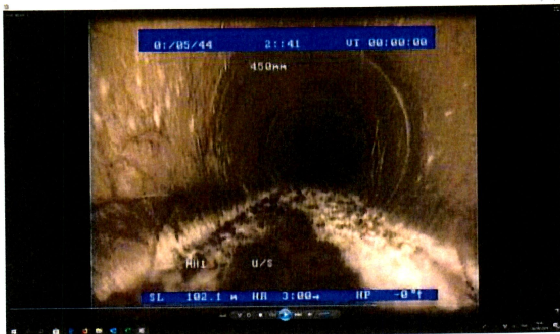
Distance 102.1m Extensive root growth. No Connections
