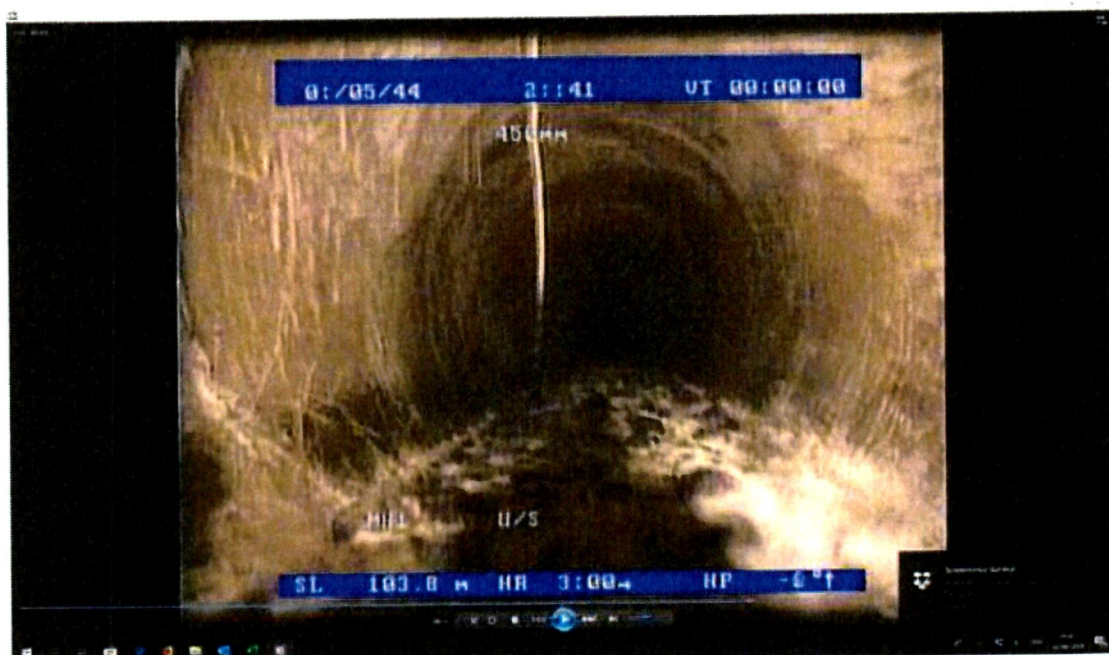
Distance 103.8m Extensive root growth. No Connections
