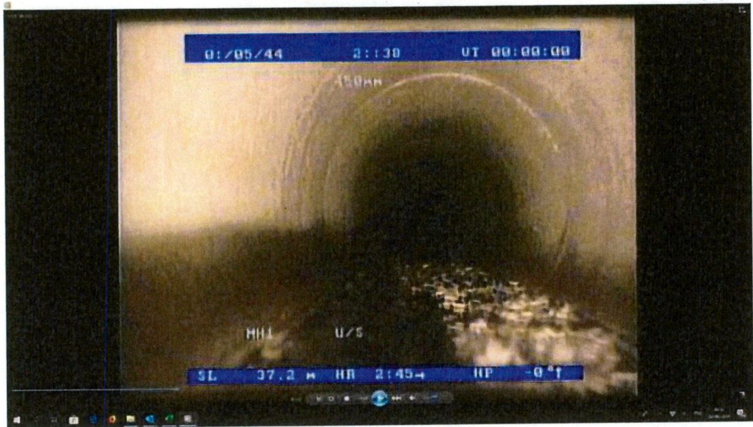
Distance 37.2m Debris in pipe. No connections
