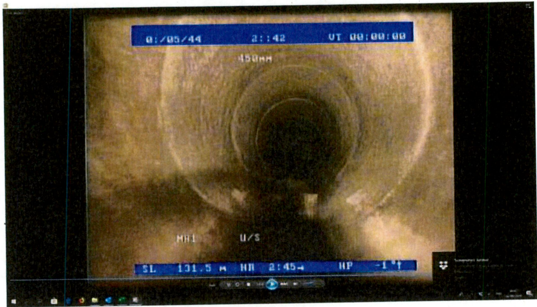
Distance 131.5m Debris in pipe. No Connections
