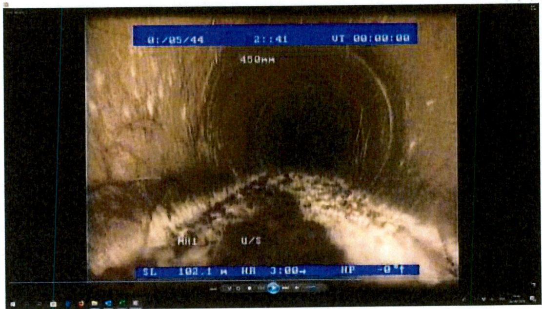
Distance 102.1m Extensive root growth. No Connections
