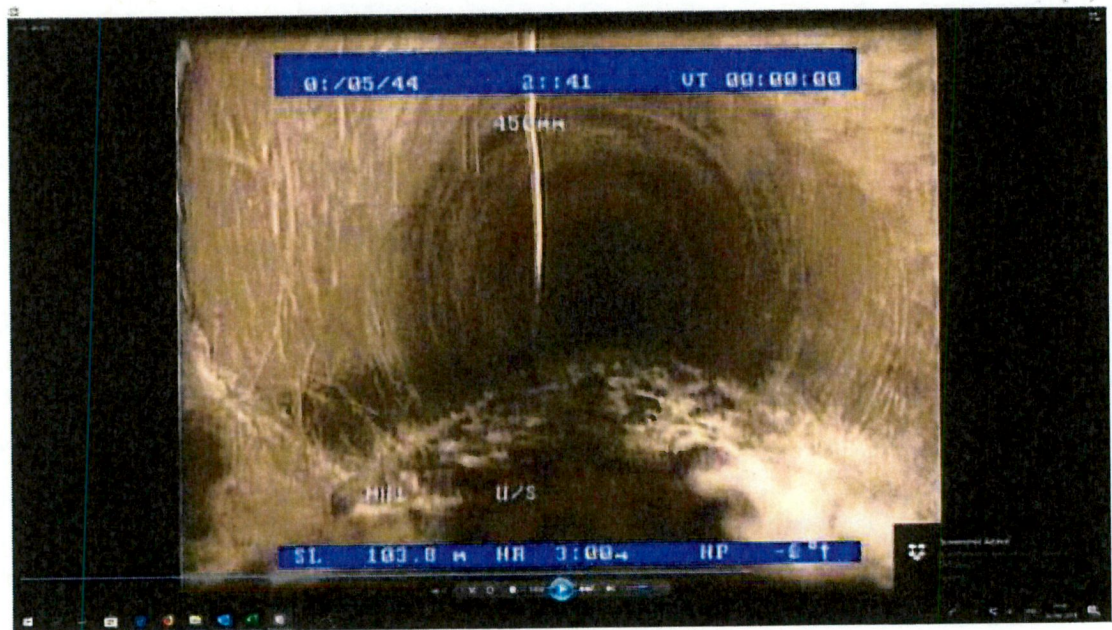
Distance 103.8m Extensive root growth. No Connections
