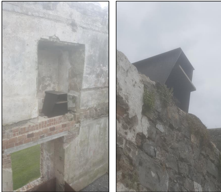
Plate 2 Barn owl boxes located in the second and third floor of the Grange Castle
