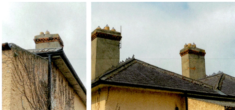
Right: Relationship between the corner extension roof and the eaves to the main house and Left, the similar relationship between the central extension asbestos roof and the main eaves.
