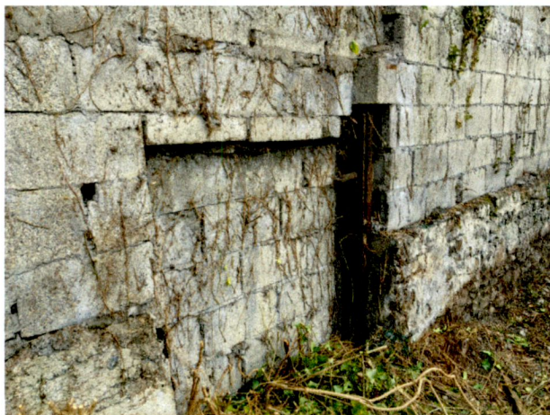
Above: The eastern site boundary wall where the proposed new entrance is proposed with a low brickwork wall lining a higher modern blockwork wall.
