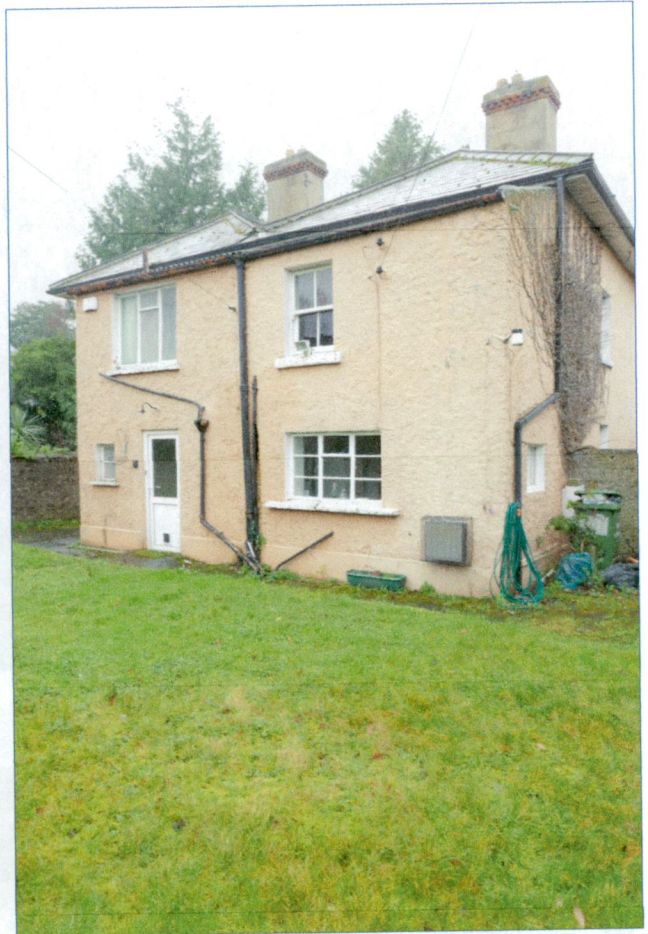
Rear (east side) of house. It is proposed to demolish the modern left half of the return and to refurbish and extend the older section.
