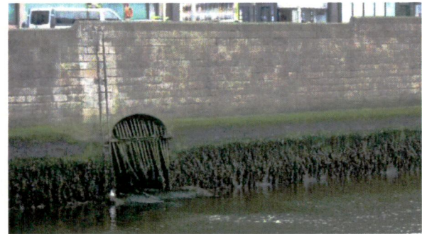
Plate B24 Stock image of the Poddle-Liffey confluence at Wellington Quay, Dublin City centre
