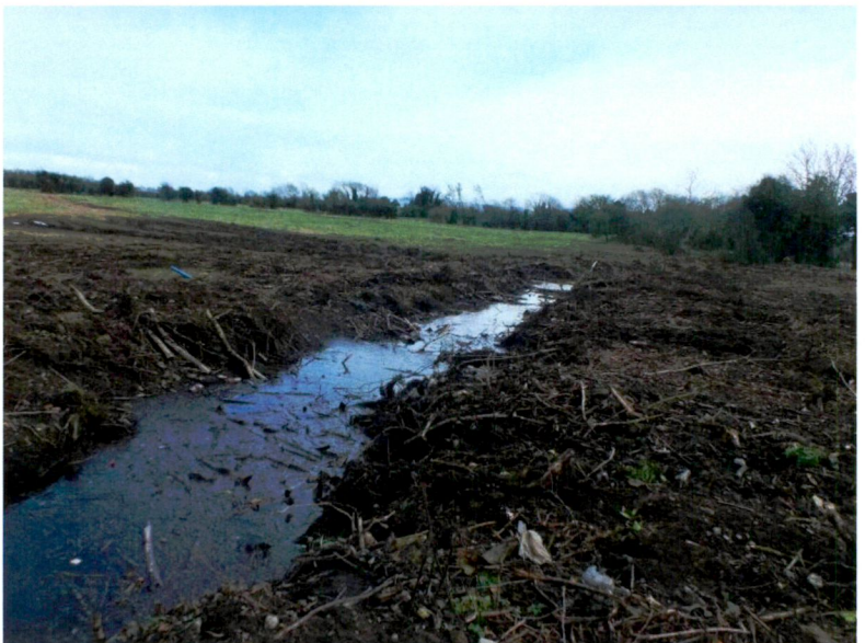
Plate 12. Hedgerow removal and scrub clearance at central north of the survey area.
