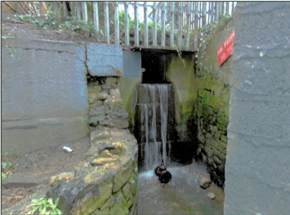
Photo 3: Concrete Tank Outlet
