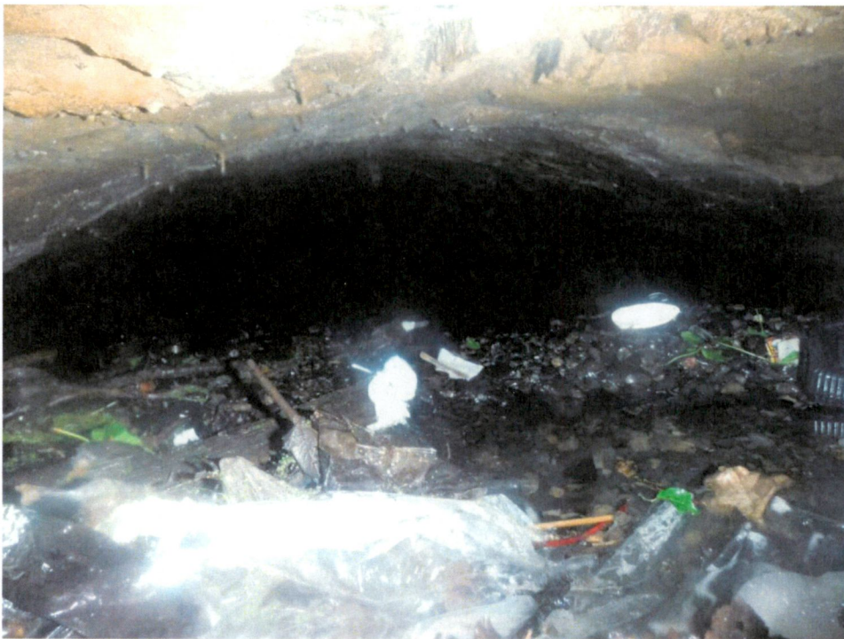
Photograph No. 2 Upstream End @ 2 m. Blockage in Arch Barrel
