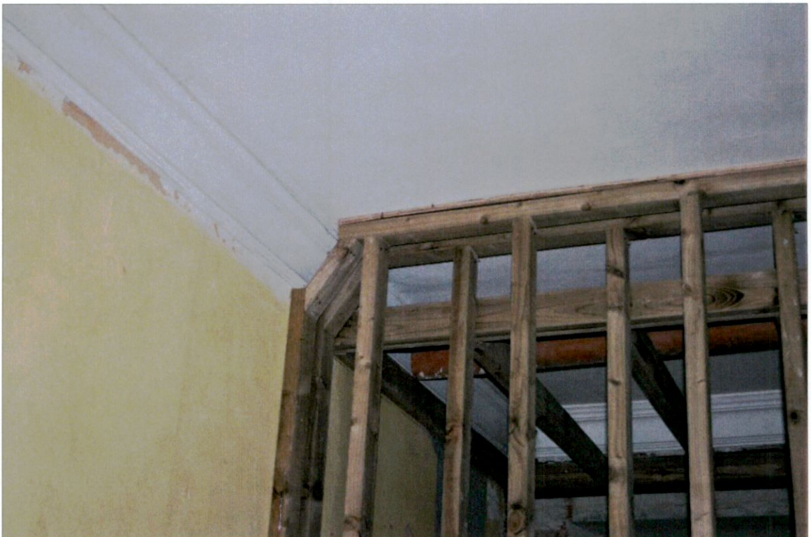
Timber-framed partition wall inserted within larger room avoiding irreversible interference with continuous moulded plaster ceiling decoration. Where possible, new proposed services should be concentrated within inserted partition walls in order to minimise chasing of original walls.
