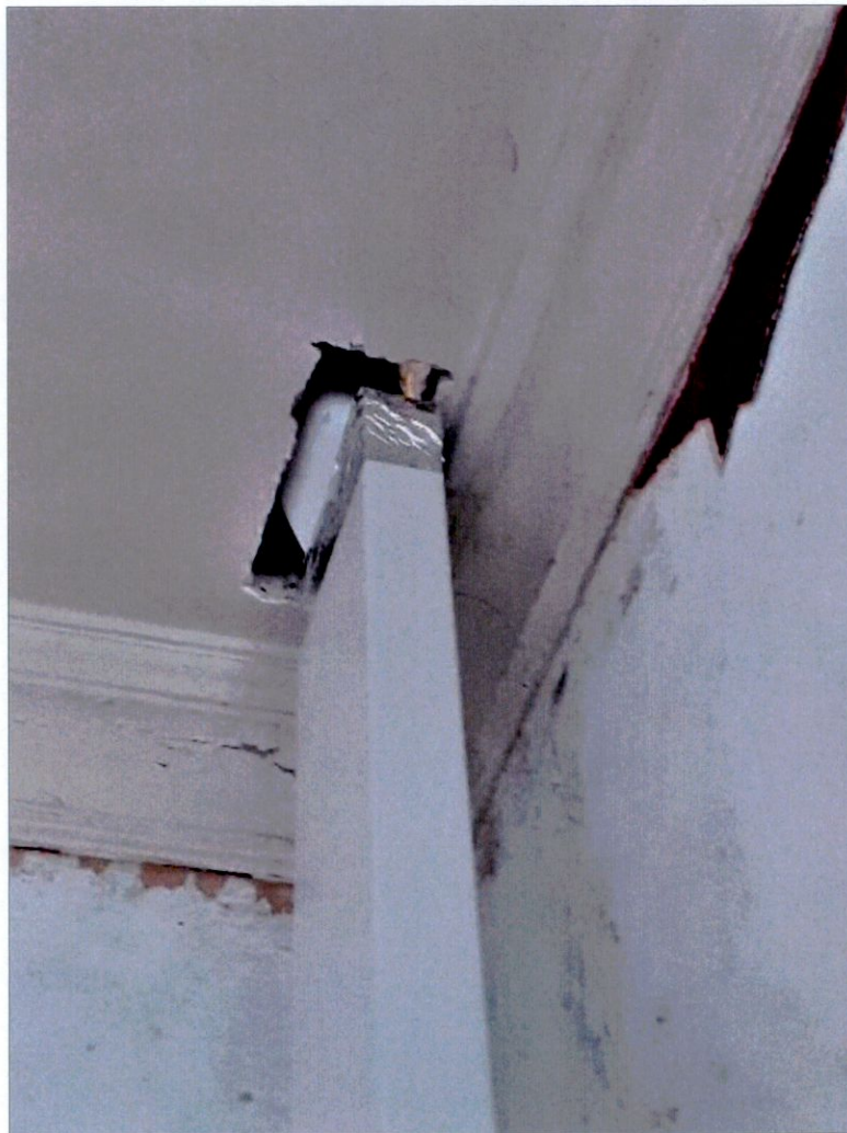
Mechanical ventilation duct converted from round to rectangular profile in order to divert around moulded plaster ceiling cornice. This duct can later be boxed-in, but no irreversible interference will be caused to significant historic plaster detail.
