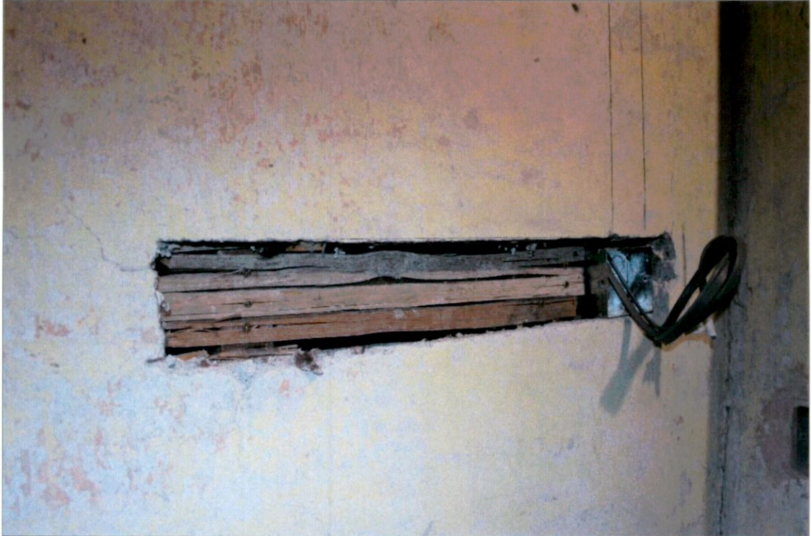
Timber ground inserted between studs on historic lath-and-plaster partition to provide adequate support for installed socket, wiring for which was fished down behind lath-and-plaster surface causing minimal interference to historic fabric which will be made good with laths and lime plaster. Unlike in the above example, all timber should be pilot-holed before it is screw-fixed.
