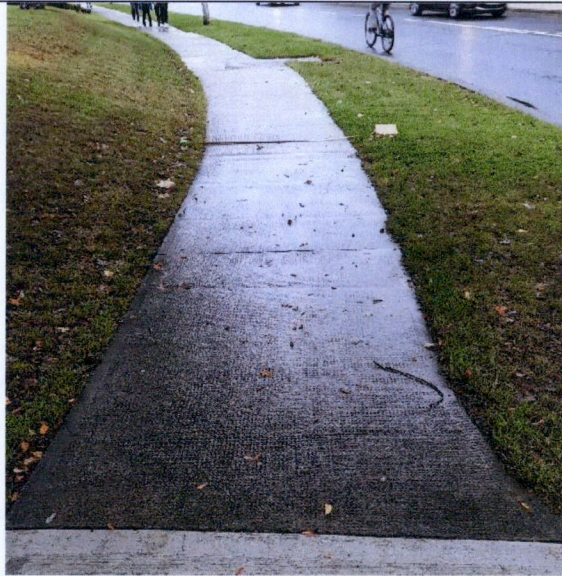
Figure 19: Widen 0.25m LHS and RHS. Chainage ~ 230.0m. Arrowed line 2m wide. Rest of path widen 0.5m to RHS
