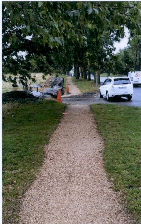
Figure 6: Widen 0.8m to RHS to avoid roots. Permeable paving under canopy. Chainage ~ 100.0m. Arrowed line 2m wide.
