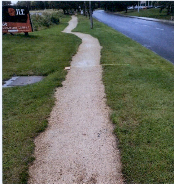
Figure 2: Widen 0.8m to right hand side (RHS) to avoid manhole. Chainage ~ 17.0m. Arrowed line 2m wide.
