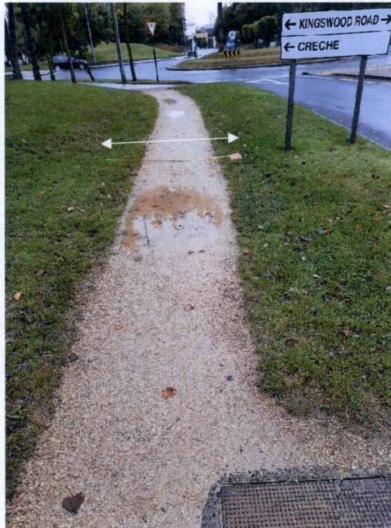
Figure 14: Widen 0.3m to LHS & RHS. 0.5m from outside of sign. Chainage ~ 203.0m. Arrowed line 2m wide.
