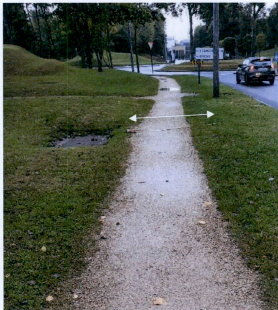
Figure 12: Widen 0.6m to RHS. Avoid manhole. Chainage ~ 190.0m. Arrowed line 2m wide.
