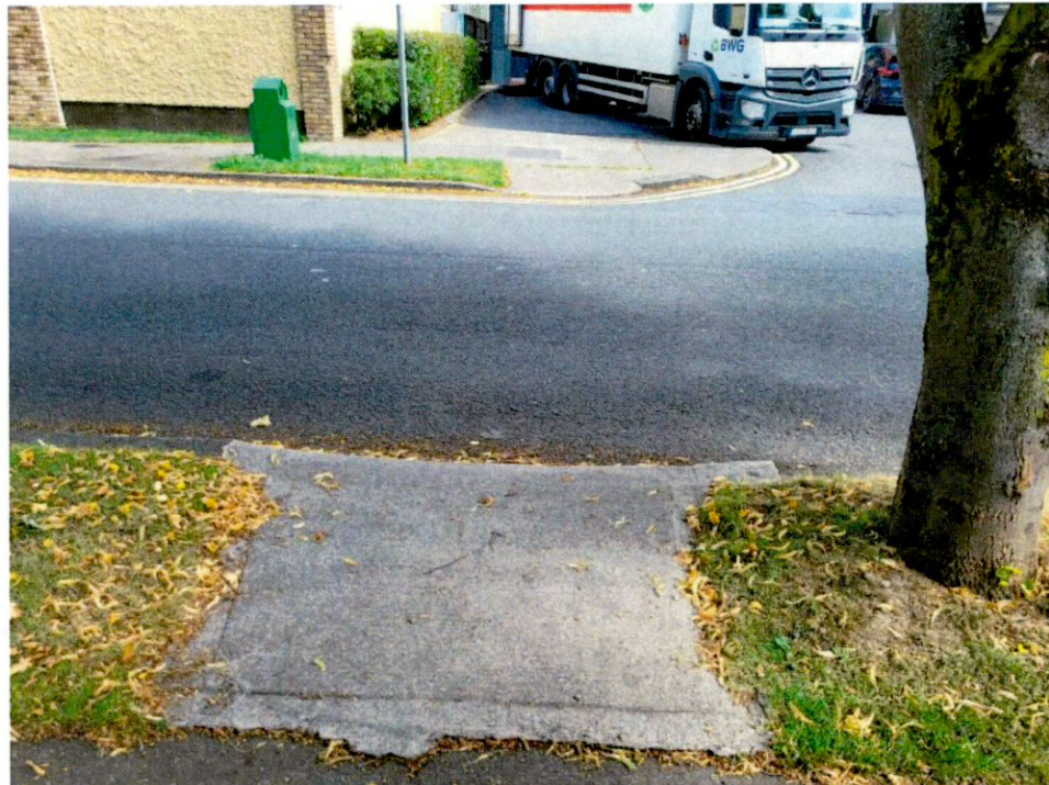
Figure 20: Narrow Crossing Point with Poor Intervisibility
