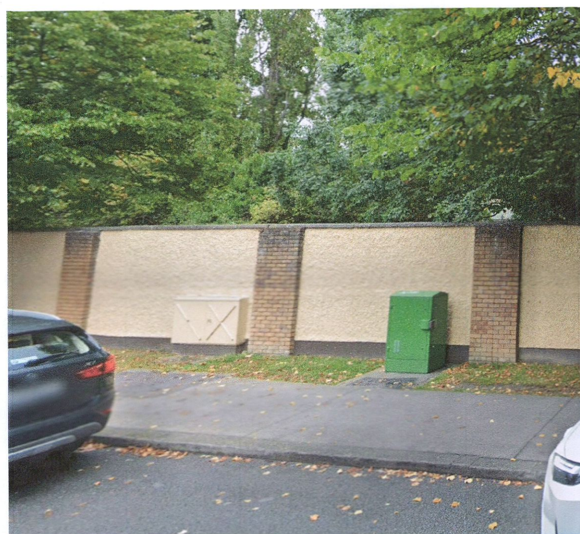
EXISTING TELECOM CABINETS TO REMAIN
