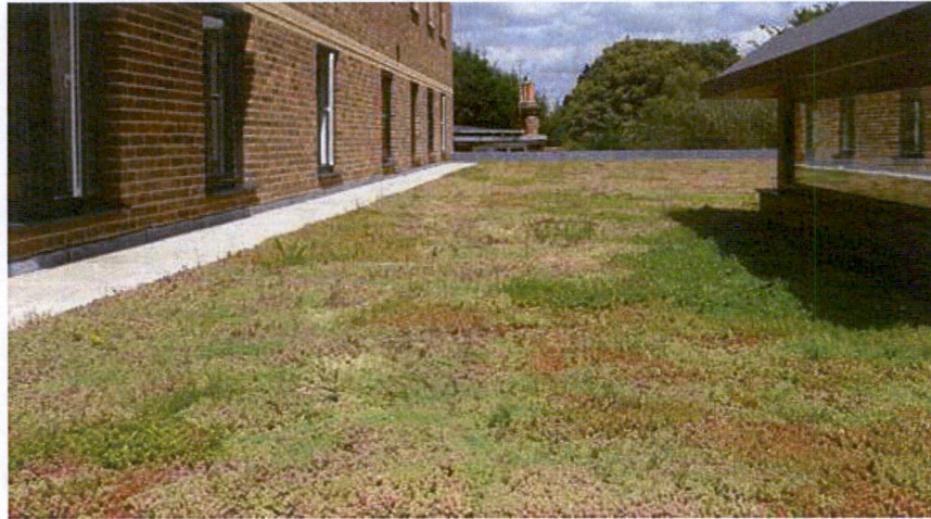
Figure 3: Sedum SuDs Roof System
