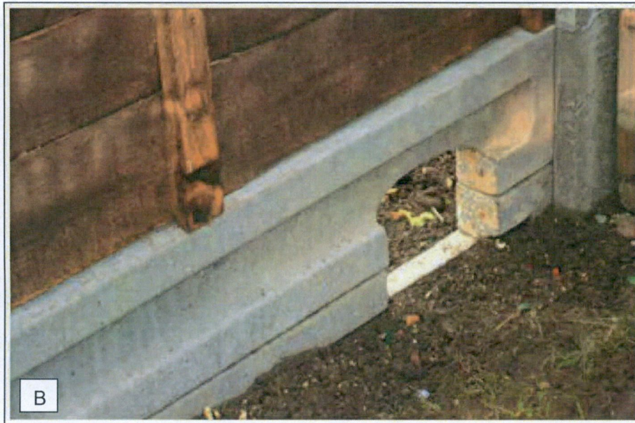
Figure 6-2: Examples of 'Hedgehog highways' that can maintain habitat connectivity for Hedgehogs in residential developments (Images: BHPS Guidance document).
