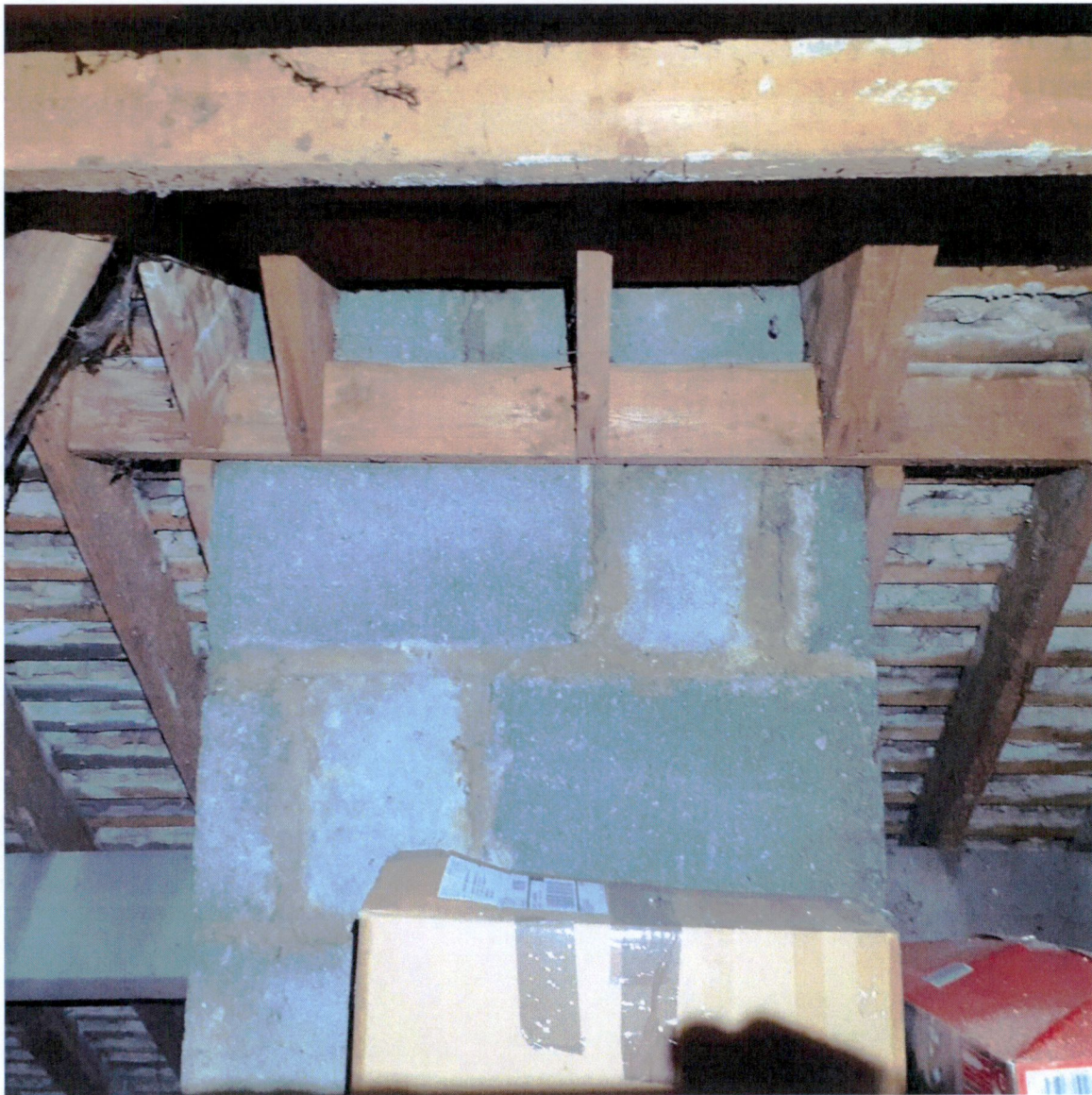
Plate 3: Chimney breast and slates with parching (no roof felt present) in attic space of dwelling.
