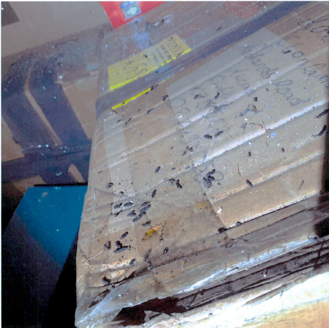
Plate 1: Bat droppings in the attic space of the dwelling.
