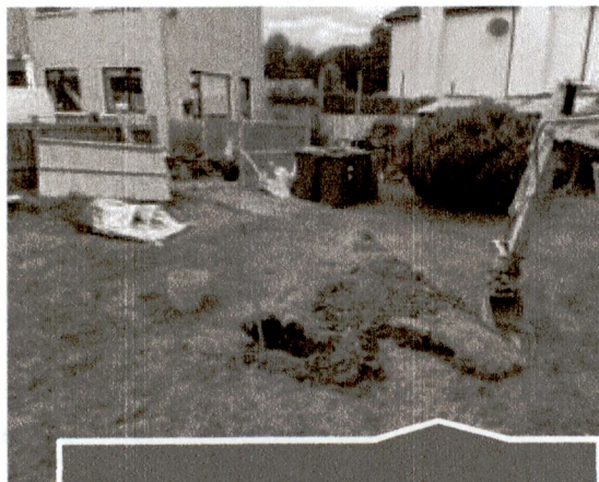
Site during testing
