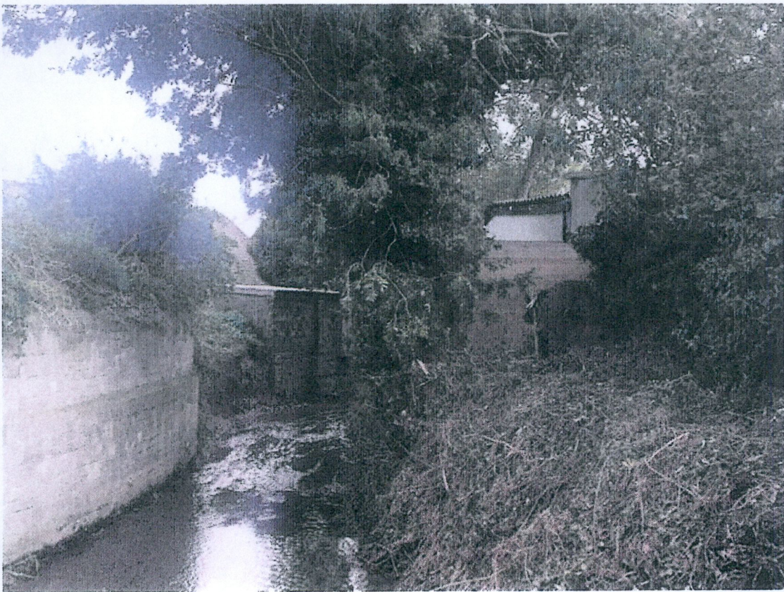
14) Cleared riverbank at the rear of no. 3 & building at edge of river opposite
