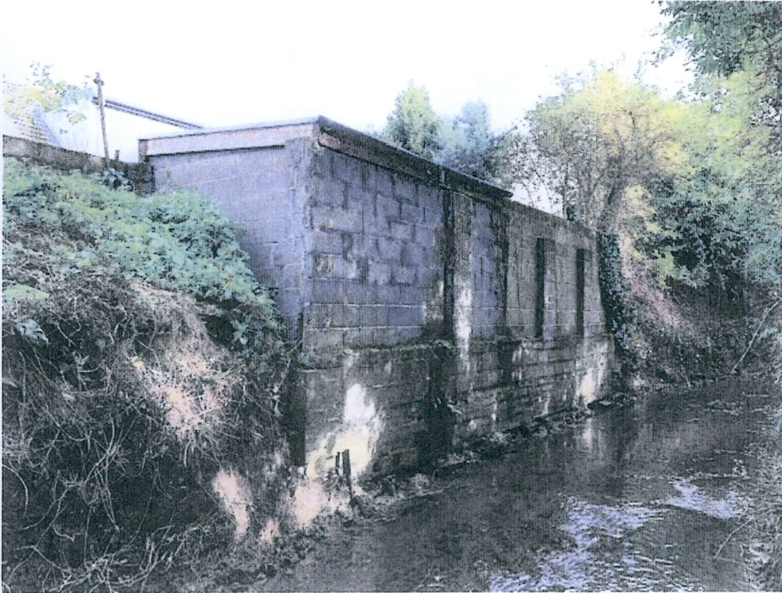
15) View of Shed built at edge of riverbank to rear of no. 38 Limekiln Road
