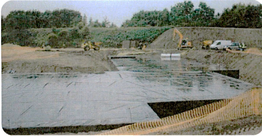
Attenuation Tank under Park and Ride Scheme showing versatility of modular system.
