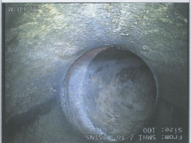
Joint displaced 25mm
