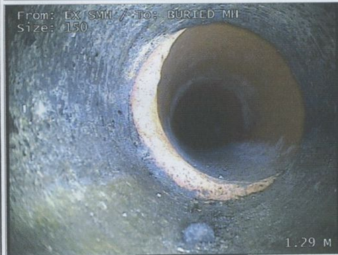
Joint displaced 15mm
