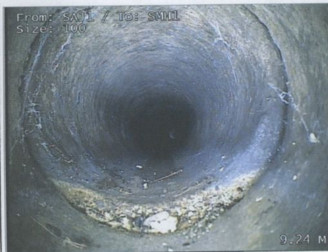
Joint displaced 10mm
