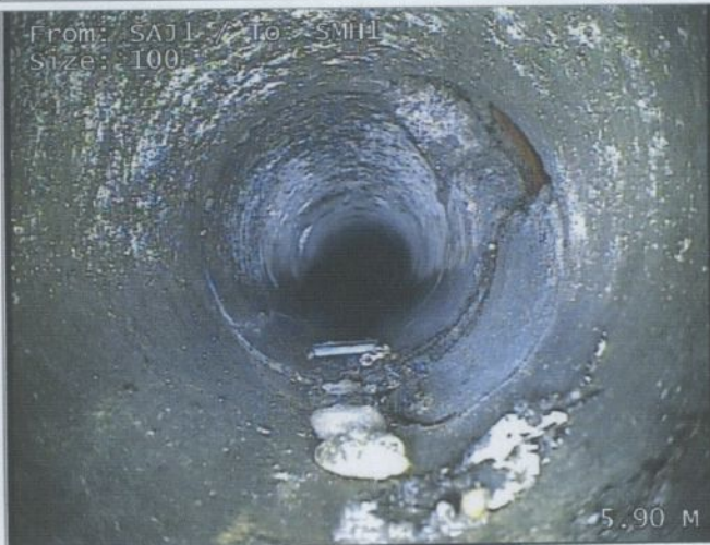
Connection defective at 1 o'clock, diameter 100mm
