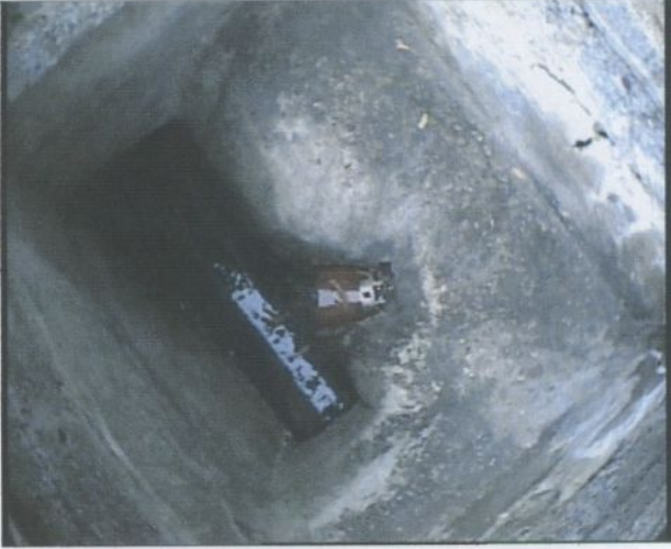
Manhole / Access Point: EX FMH Internal
