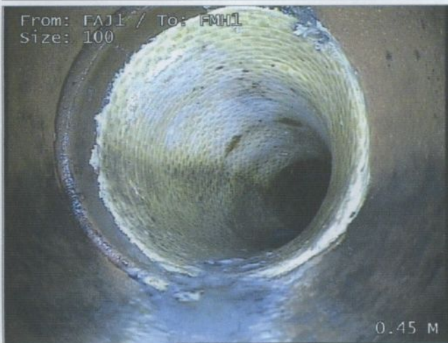
Line of drain/sewer deviates right
