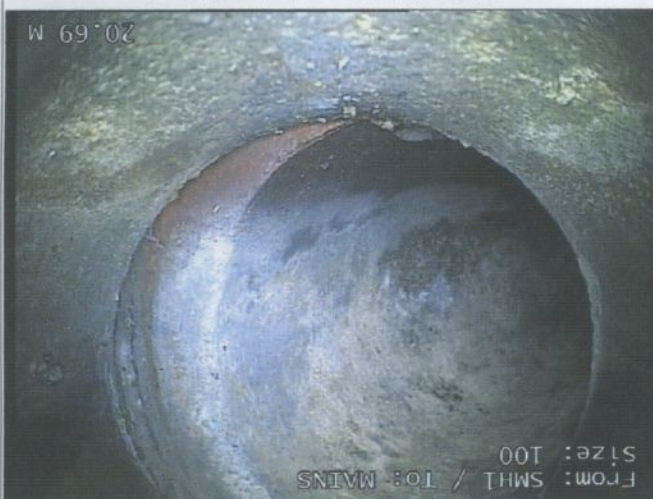
Line of drain/ sewer deviates left
