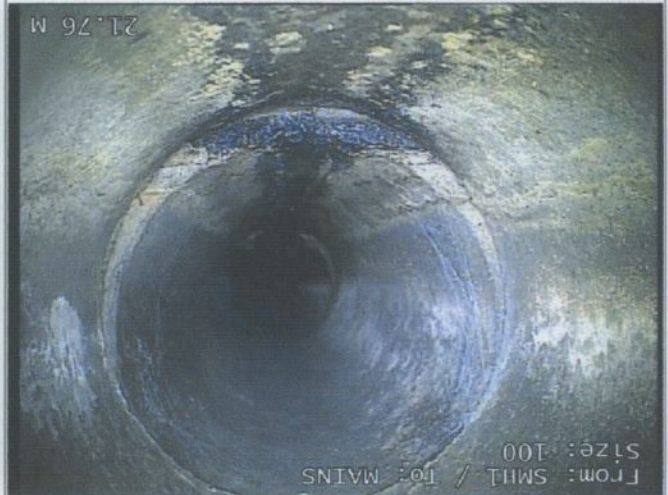
Joint displaced 10mm
