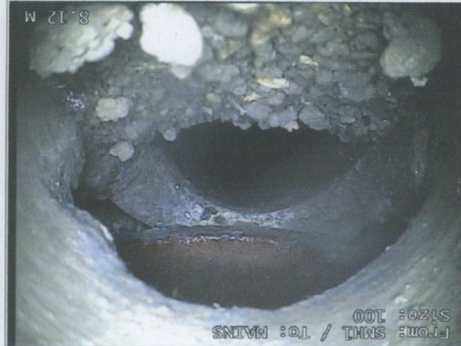
Connection defective at 12 o'clock, diameter 100mm
