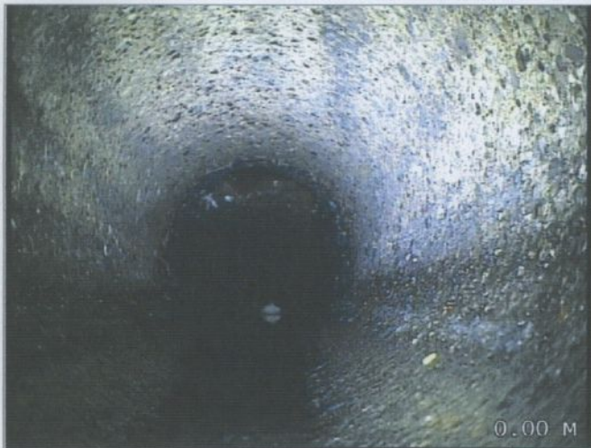
Start node type, manhole, reference EX FMH
