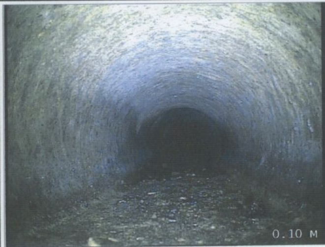
Start node type, inspection chamber, reference SAJ1
