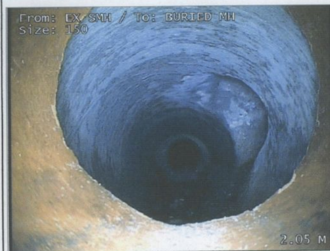
Joint displaced 15mm
