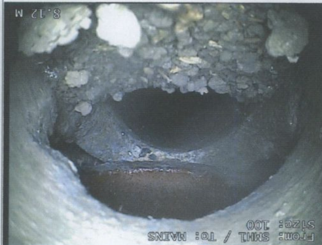
Settled deposits hard or compacted 75% cross-sectional area loss
