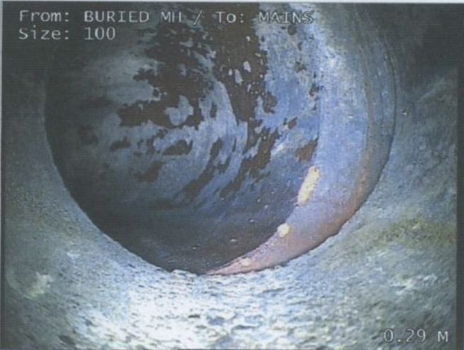
Joint displaced 20mm
