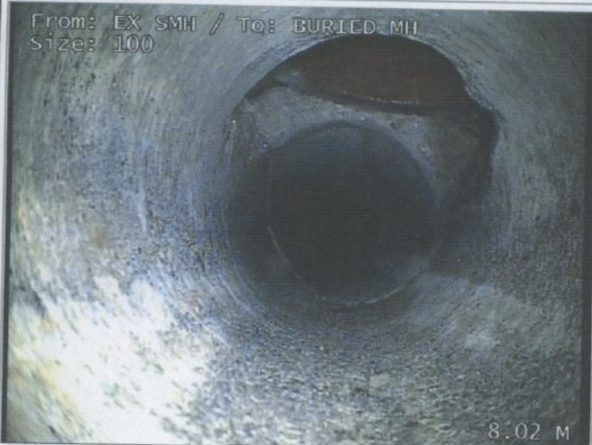
Connection defective at 12 o'clock, diameter 100mm
