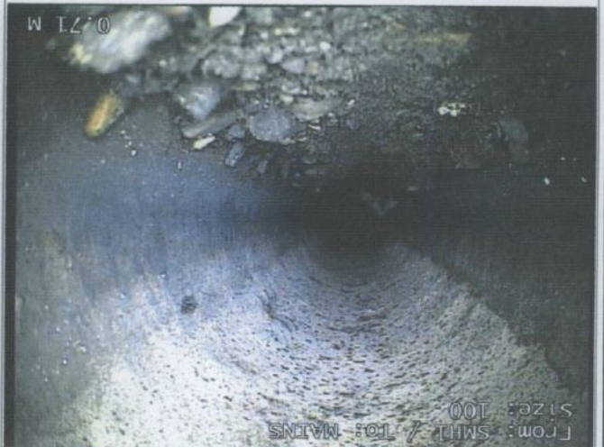
Settled deposits coarse 25% cross-sectional area loss
