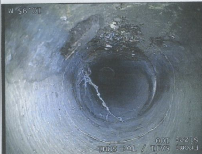
Crack circumferential from 7 to 4 o'clock
