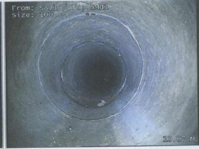
Crack circumferential from 12 to 12 o'clock
