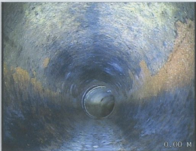
Start node type, inspection chamber, reference FAJ1
