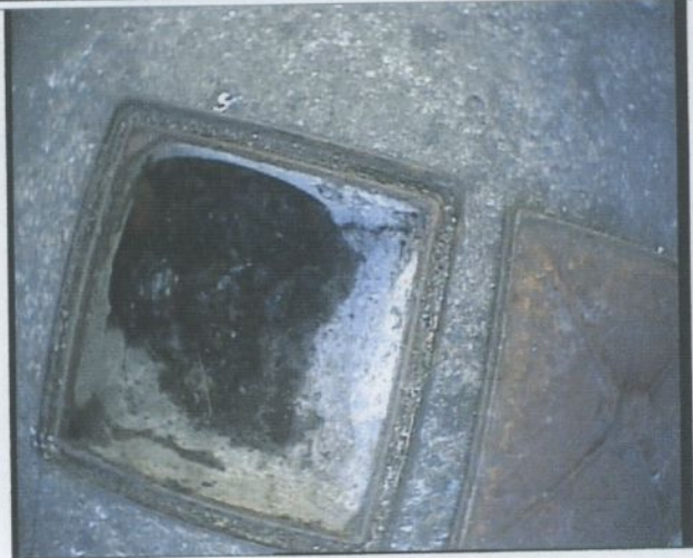
Manhole / Access Point: SAJ1 Internal
