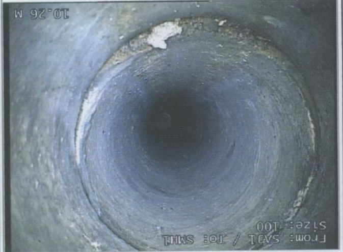
Joint displaced 10mm
