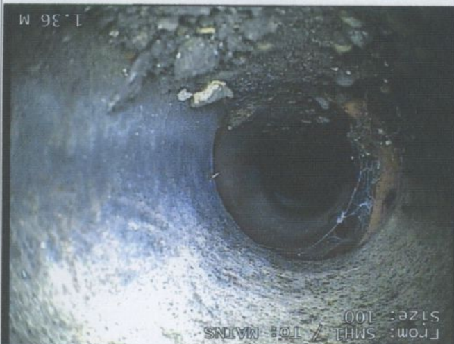
Joint displaced 15mm
