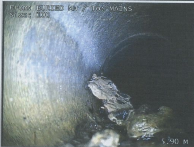
Settled deposits coarse 25% cross-sectional area loss - Remark: STONE IN LINE
