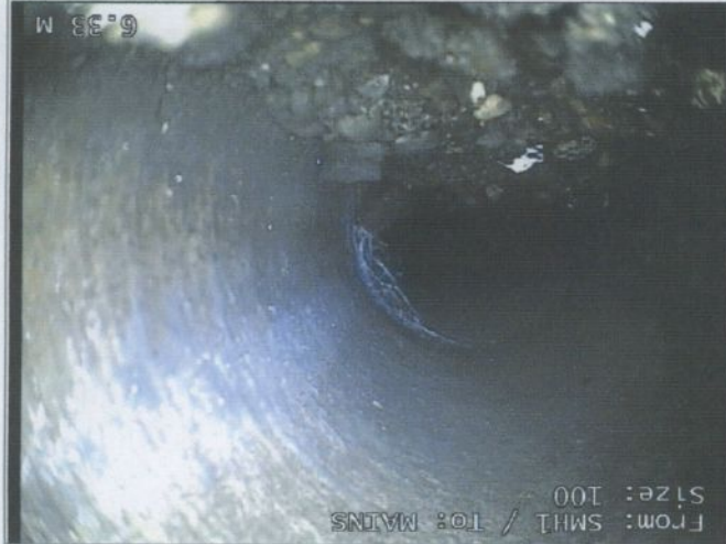
Settled deposits hard or compacted 40% cross-sectional area loss
