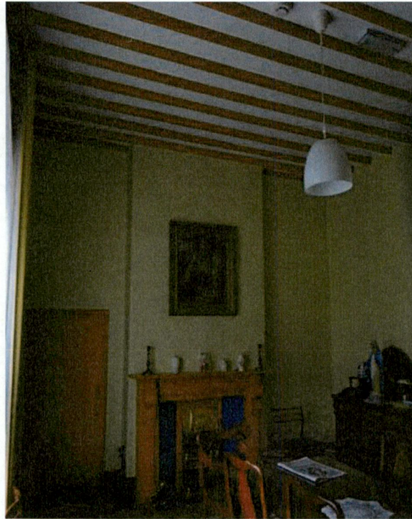
View G5 above of the second reception or parlour off the entrance hallway with exposed joists and matching chimneypiece. View below G6 of the original window casing with panelled shutters exhibiting chamfer detail and original sliding sash windows.
