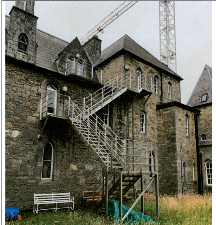
Fig 17: The existing external staircase is to be removed and the new stair tower 02 located on the footprint of the existing metal staircase.
