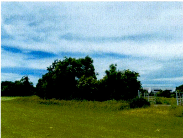
Above image shows the concrete bridge providing access to the adjoining field at the northern end of Hedge No.2.
