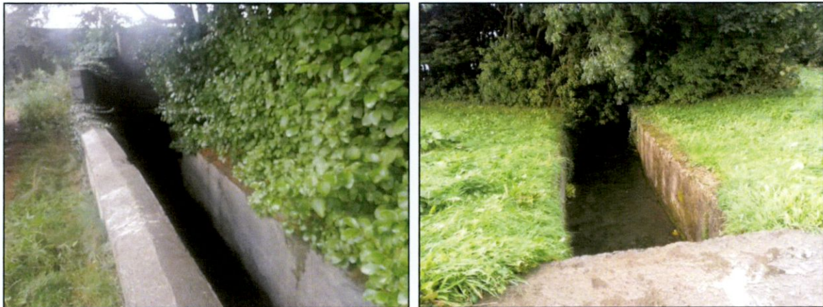
FIGURE 4. GREENOGE STREAM AS IT BRIEFLY OPENS BEFORE FLOWING UNDER N7, AND AS IT EMERGES FROM CULVERT NORTH OF N7.
