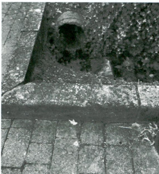
Fresh water conveyance outlet discharging to roadside ditch
