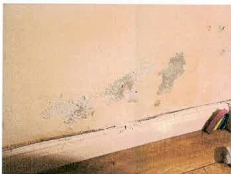
Sample of Rising Damp
