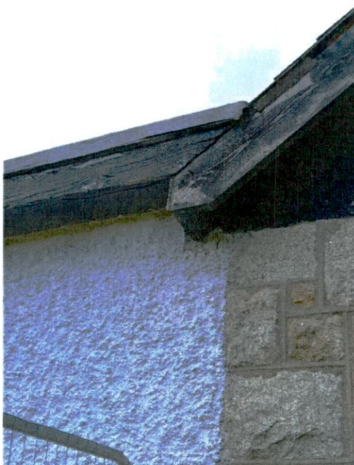
-Example of maintenance required to facias
