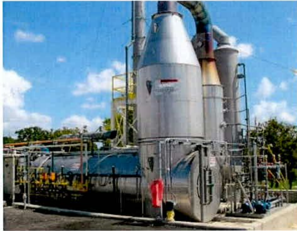
Example of a (TO) thermal oxidiser VOC abatement system
