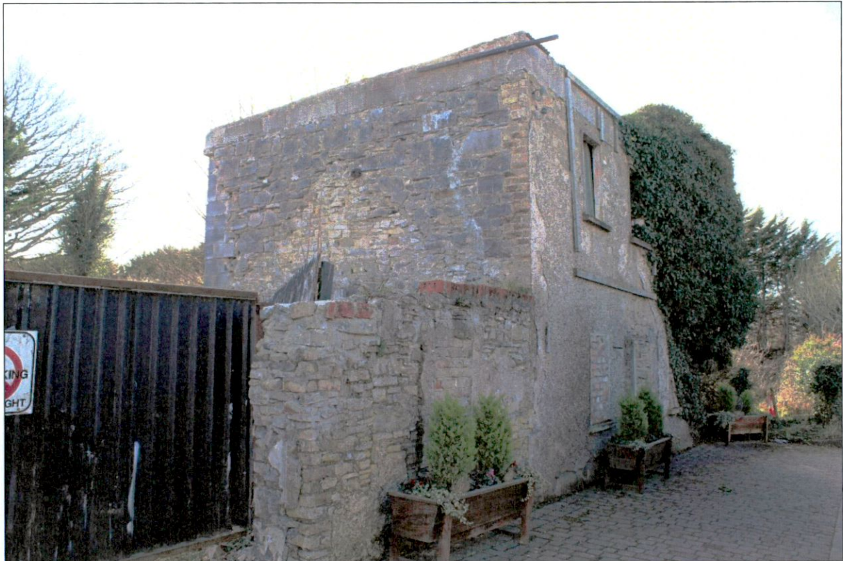
Plate 3: North façade and east elevation of former two-storey townhouse proposed to be refurbished and extended as a retail premises.
