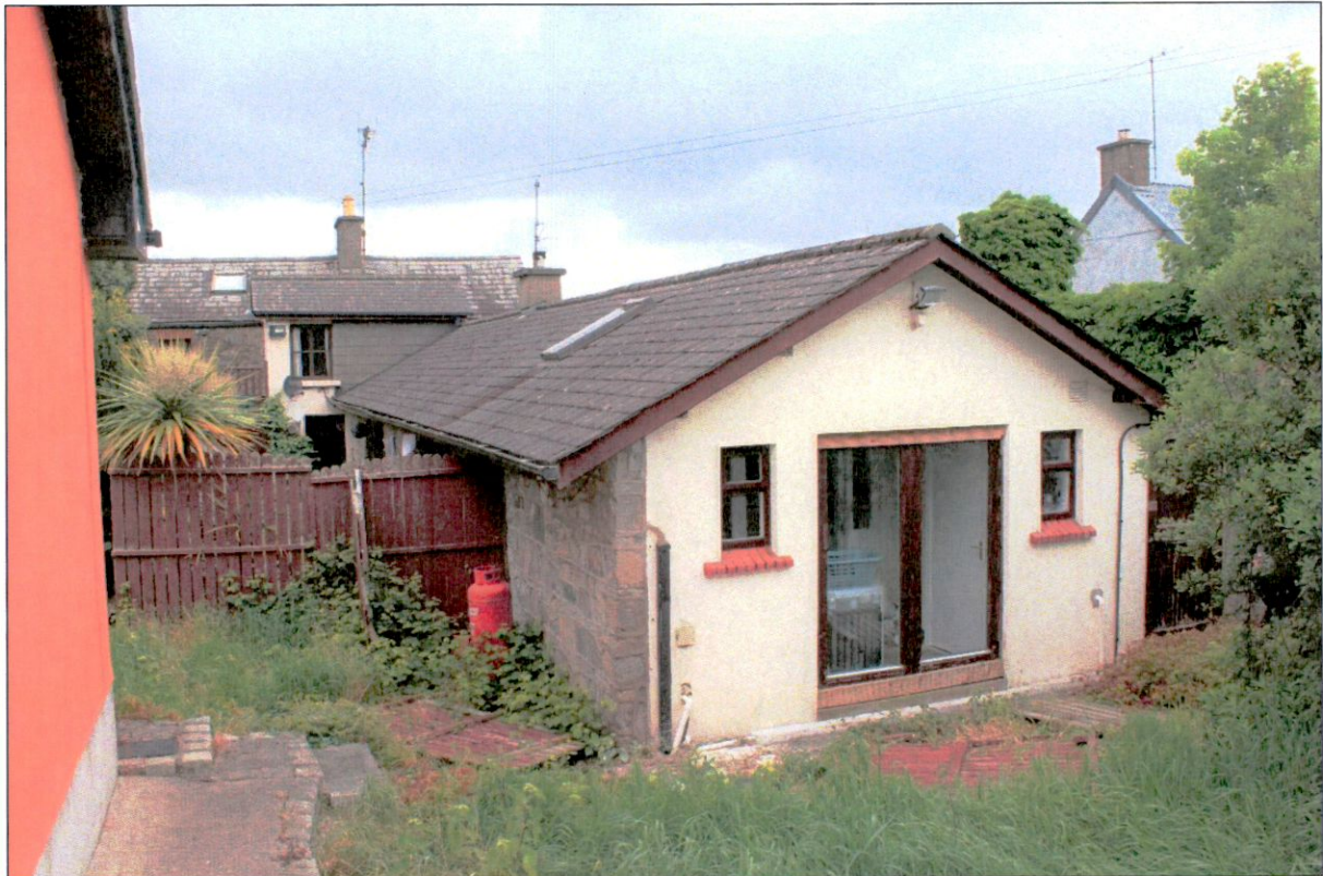
Plate 11: Modern south end of rear extension to Kelly Estates proposed to be truncated back approximately to where existing timber fence is located. Fence to be replaced with new 2m boundary wall.
