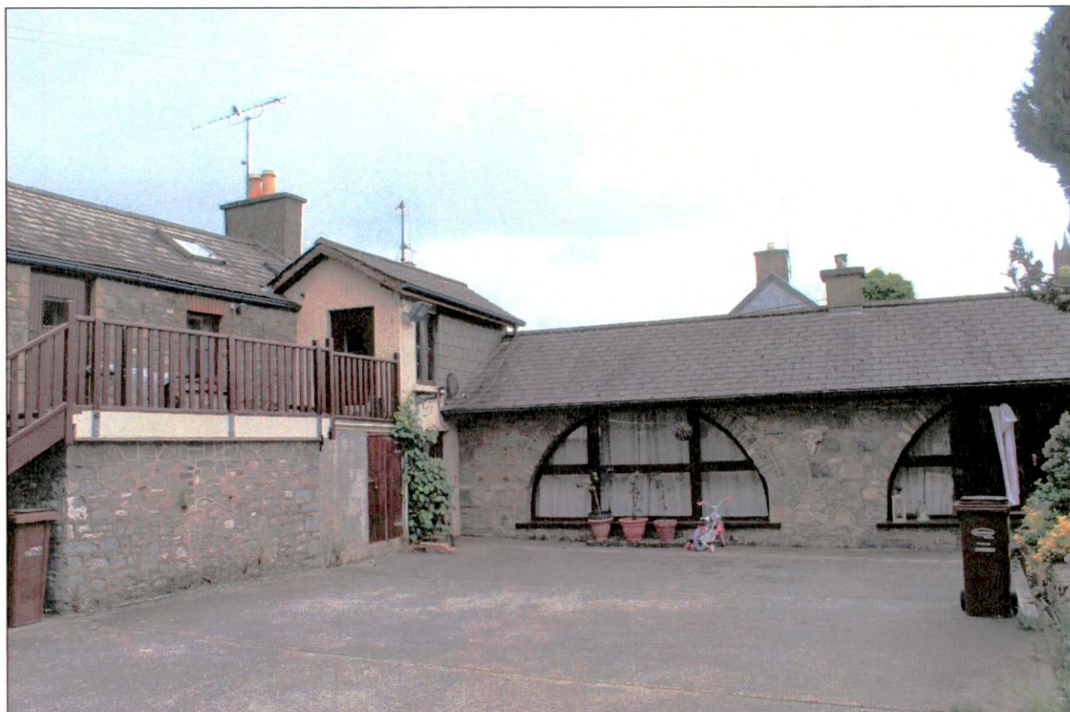
Plate 10: West elevation of existing rear extension to Kelly Estates building to be truncated approximately along right edge of photograph.
