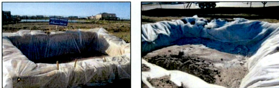
Figure 5.13.1; Example of a simple lined concrete washout skip.
