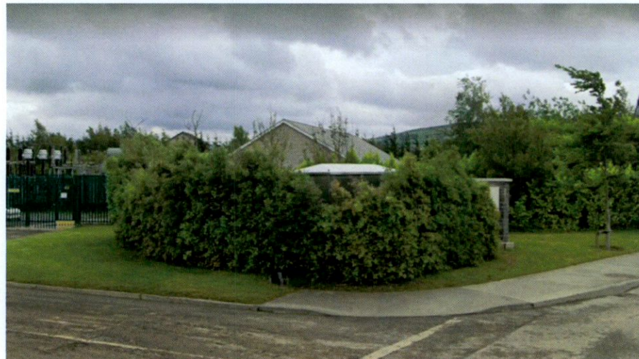
Picture 22: View of existing substation from Citywest Village Avenue – Source Google Maps
