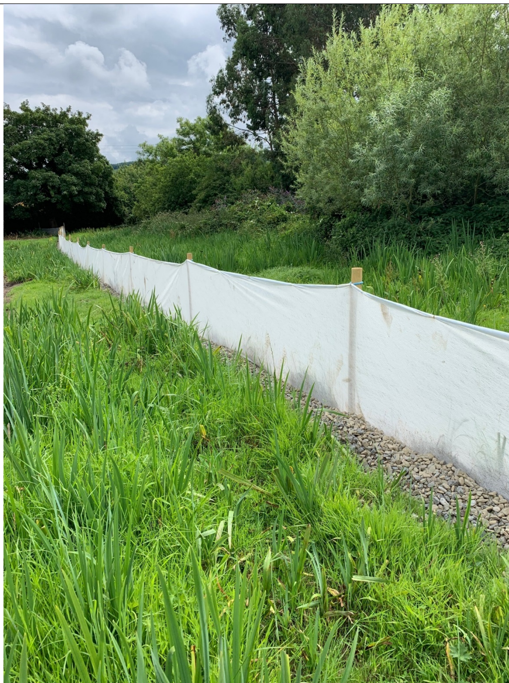
Silt fencing, continuous and complete to the site boundary and including the field edge drain,
