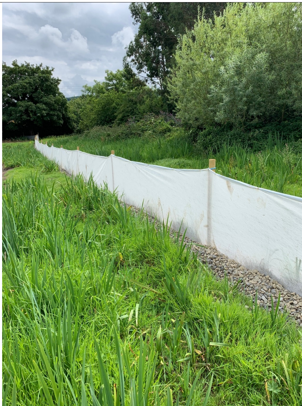
Silt fencing installed at a set back from the river. Trench and gravel correctly laid as per the specification
