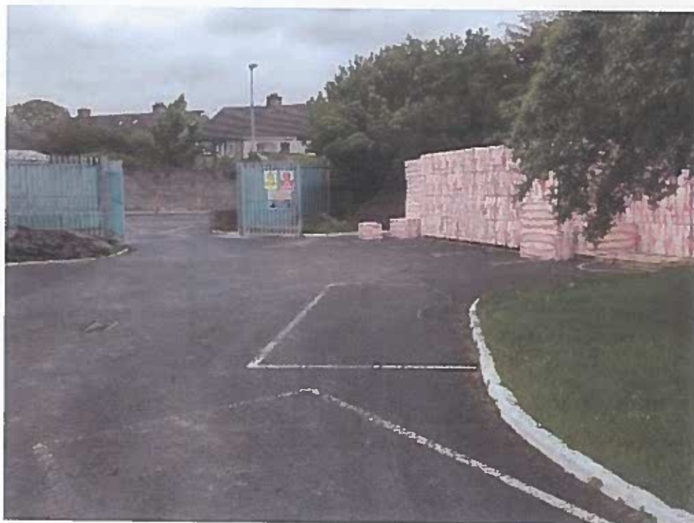
Photo 4: 23-07-22 Cavity Wall Insulation stock piled on site reducing risks associated with material supply and lead in times.
