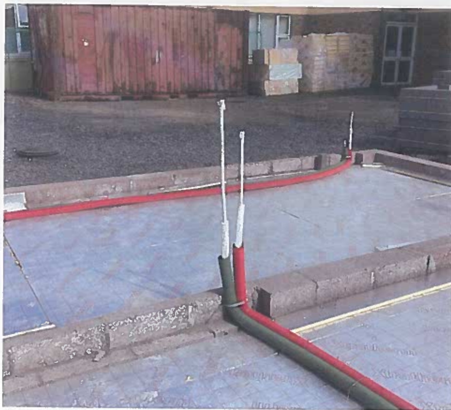
Photo 3: 23-07-22 – Radon, insulation, and pipework complete ready for ground floor slab pour scheduled for week starting 25 th July 2022
