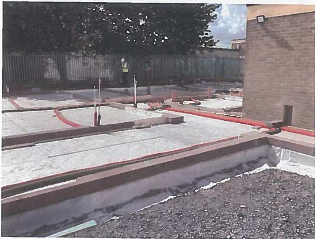
Photo 2: 23-07-22 – Radon, insulation, and pipework complete ready for ground floor slab pour scheduled for week starting 25 th July 2022
