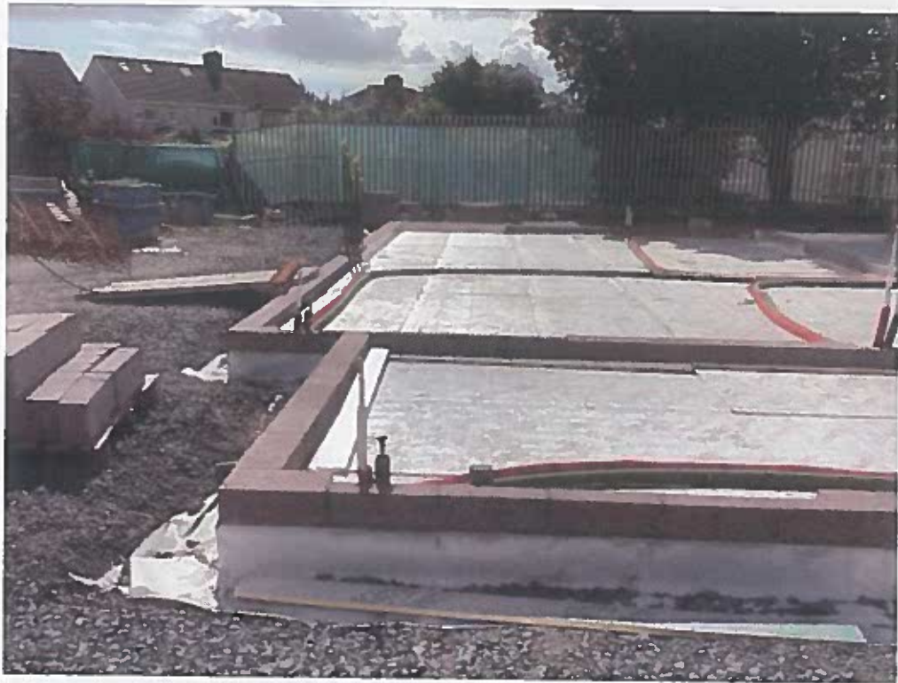
Photo 1: 23-07-22 – Radon, insulation, and pipework complete ready for ground floor slab pour scheduled for week starting 25 th July 2022
