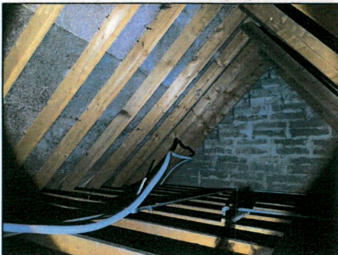
Plate 8 Attic space of building where works are ongoing. The attic has been cleared and works seemed to include refurbishing and reinsulating the area.
